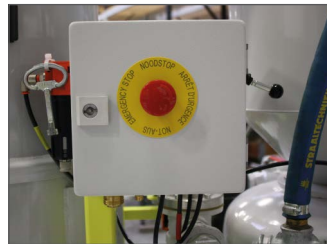
Pneumatic operated control system with anti-static tubing
